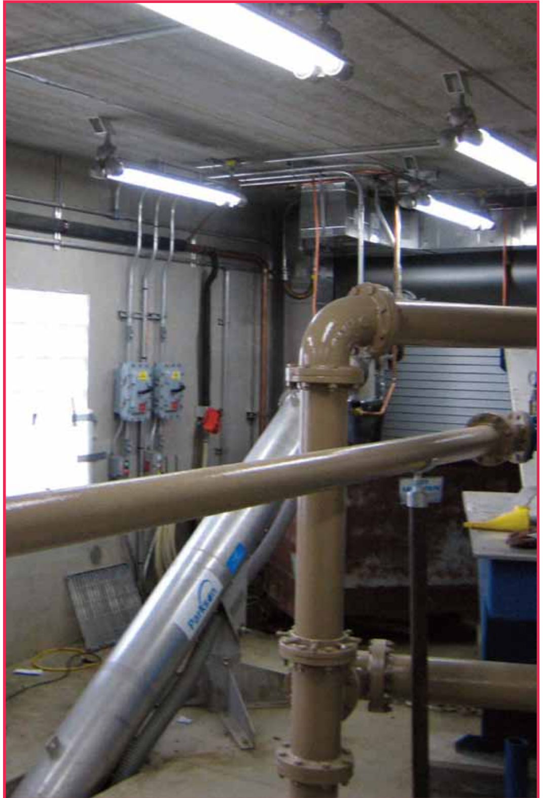
Stuart Wastewater Treatment Facility
